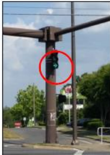
Figure 7 – No Backplates for EB/WB Right-Turn Signals
