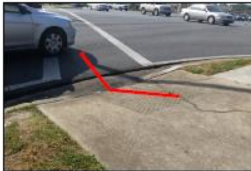
Figure 5 – At SE Corner - Change in Grade at ADA Ramp
