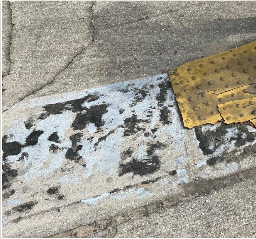
Damaged/Missing Detectable Warning Surface
