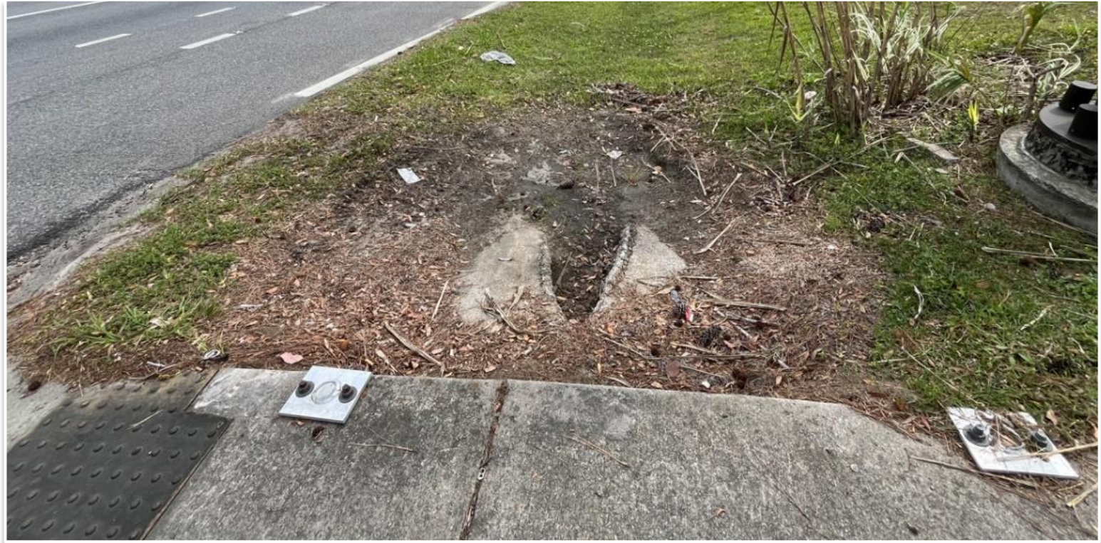
Damaged/Missing Pedestrian Safety Features (No Railing)
