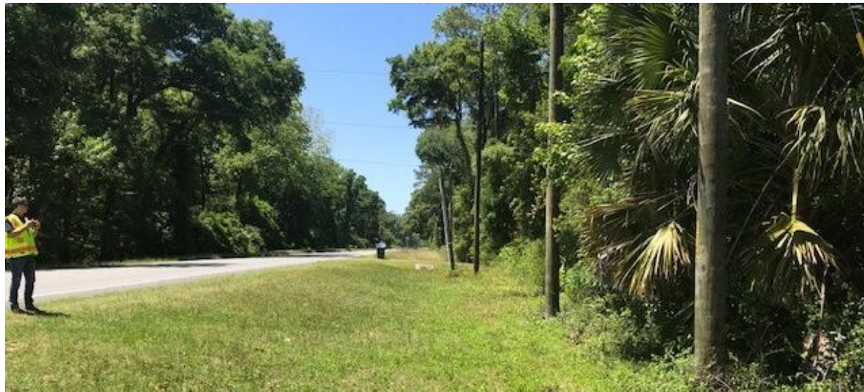
Figure 16: Overhead Electric Distribution Lines (Poles)
