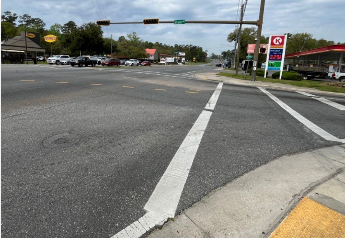
Crosswalk Without High Emphasis Markings
