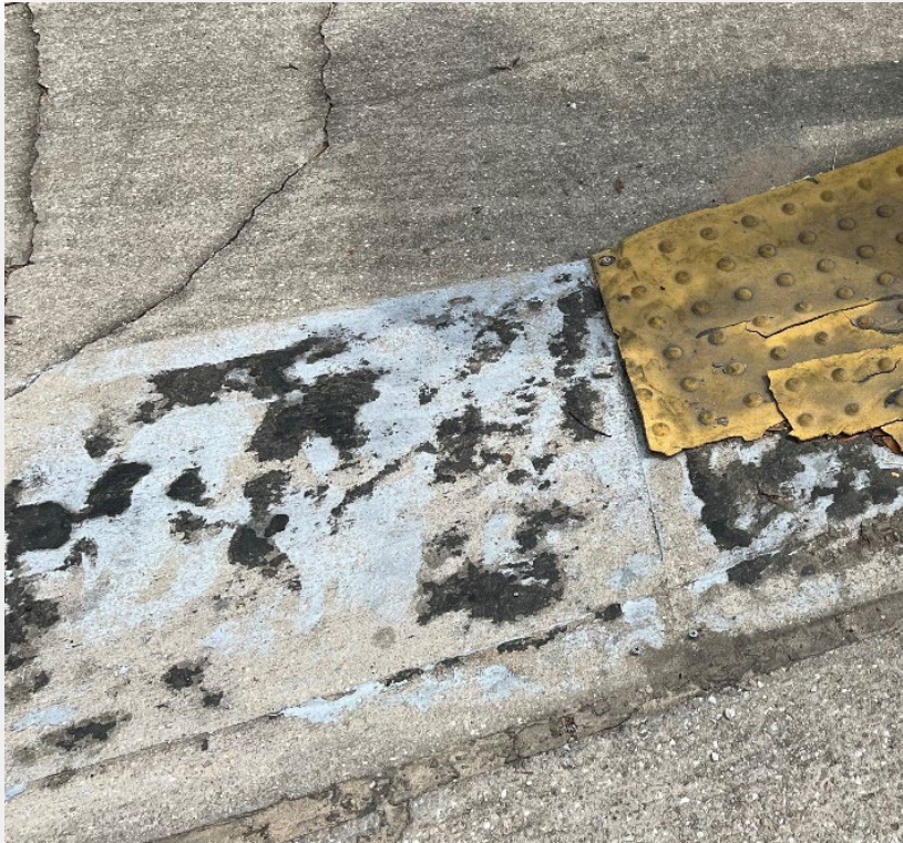
Damaged/Missing Detectable Warning Surface
