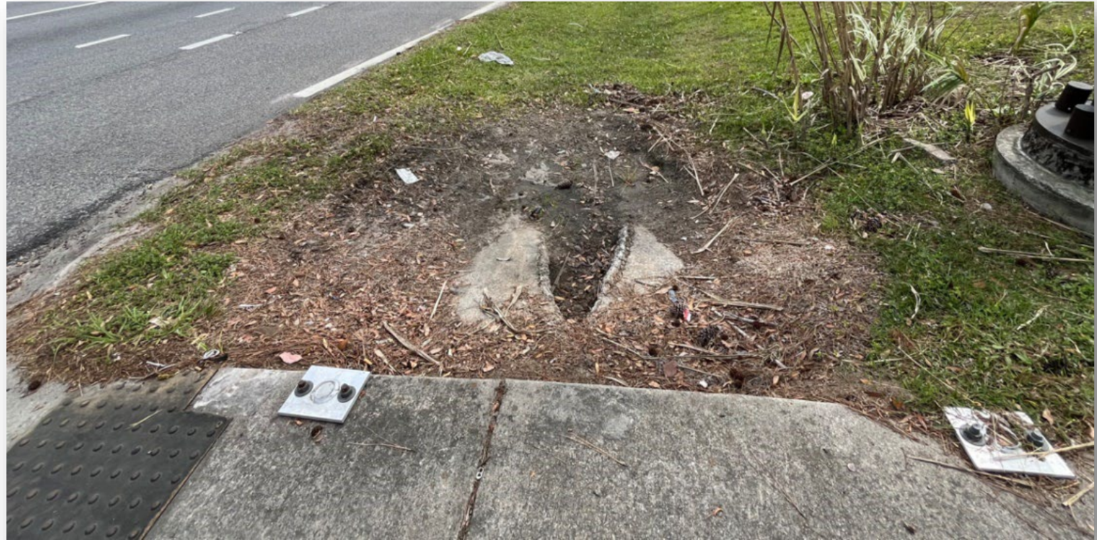
Damaged/Missing Pedestrian Safety Features (No Railing)
